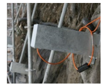
Rock anchor monitoring
