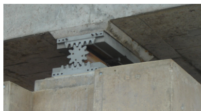
An existing roller bearing before replacement by a RESTON®POT bearing, supervised by mageba
