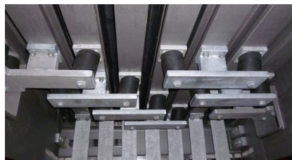
The underside of one of the expansion joints, showing its gap width control system
