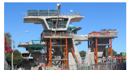
The South Road Superway under construction at Kateena Street and South Road Intersection
