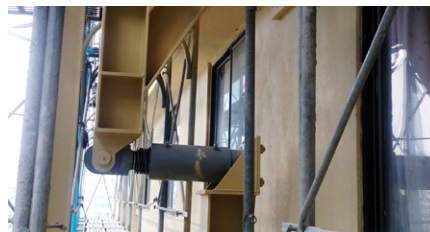
A RESTON®SA shock absorber as installed at one location in the specially constructed frame around the building
