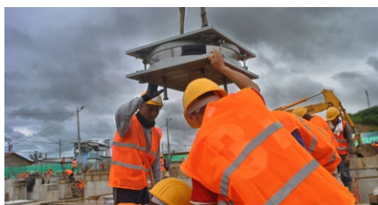
Lifting into position of a RESTON®PENDULUM seismic isolator during the construction of Muisne Hospital
