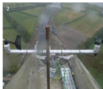
1 Presentation of measured data on web interface 2 Wind sensor as installed on the top of the pylon
