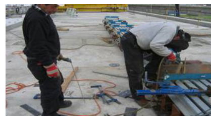
Welding together of two sections of an LR5 expansion joint on site
