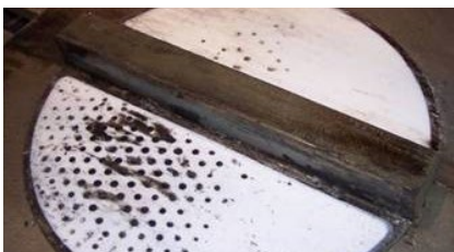
Rapid wear of PTFE sliding discs of the bridge deck's support bearings required explanation
