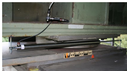
A longitudinal movement measuring sensor as installed at one of the deck's support bearings
