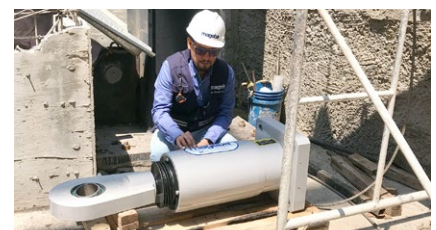
One of the dampers before installation
