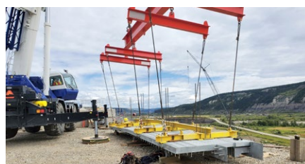
Finger joint prepared for lifting and installation into the block out at the abutment
