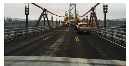
Temporary plates at the point of future installation of the expansion joints
