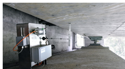
Temperature, displacement sensors and LoRa data logger at the north abutment
