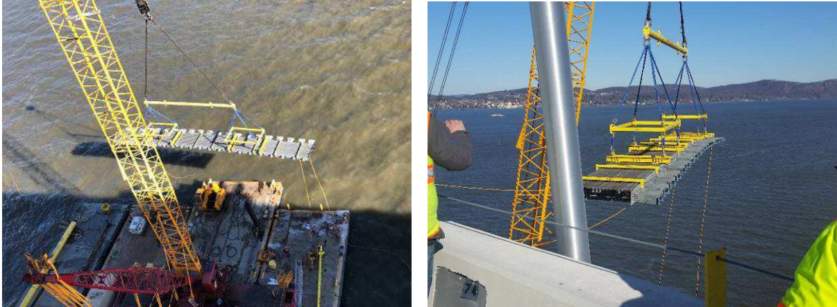
Figure 8. Lifting of an 18-gap Tensa-Modular expansion joint (29 m long, 3.5 m wide and weighing 57,000 kg) onto the bridge deck from a barge on the river 49 m below, using a floating crane
