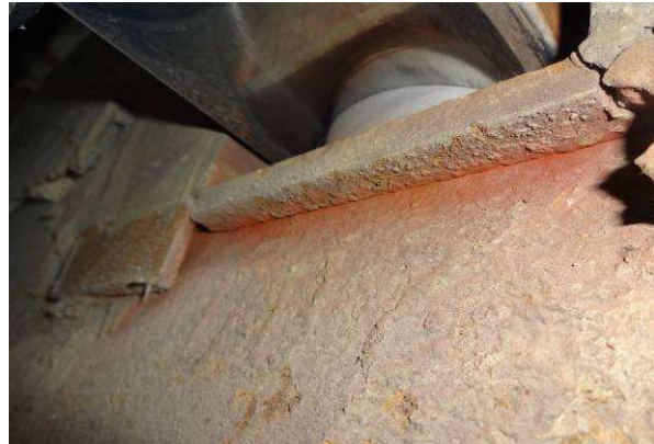
Figure 10: An example of a poorly executed connection, resulting in cracking of the structure beneath a modular joint's support bar where it enters the main structure
