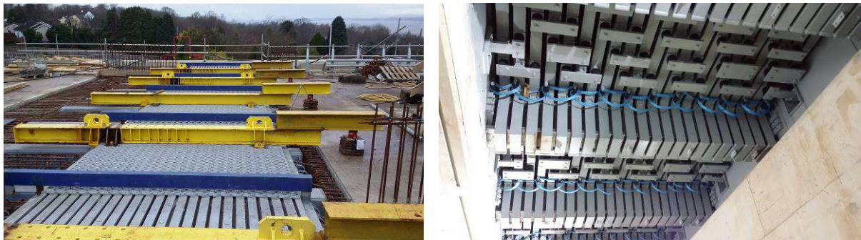
Figure 13. Adjustment of pre-setting of a 23-gap Tensa-Modular joint (length 17 m, width 5 m and weight 55,000 kg) on the Queensferry Bridge, Scotland (left), and view from below (right)
