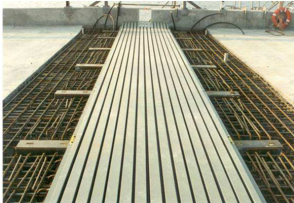
Figure 9: Connection to the main structure by concreting allows a great deal of tolerance in positioning, and an orthogonal expansion joint design can greatly simplify placing of rebar
