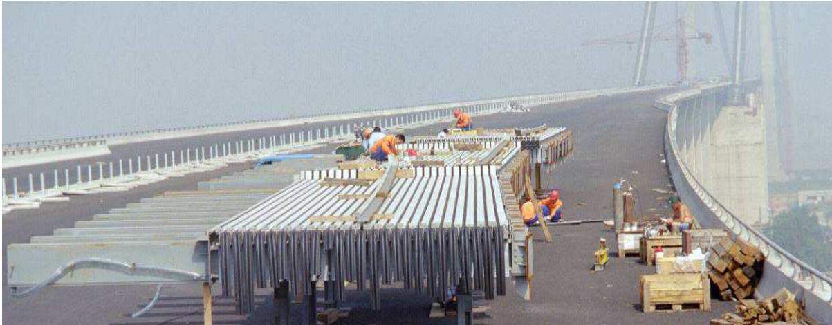
Figure 4. Assembly of the Run Yang – Nan Cha Bridge's 27-gap Tensa-Modular joints was carried out on the bridge deck, greatly simplifying transportation to site
