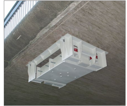
Tuned mass damper with a natural frequency of 4.3 Hz and a mass of 3.5 t, installed on a bridge in Kiel, Germany
