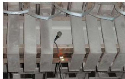
Fault simulation on a large modular expansion joint of the Taizhou Bridge. One of the steel stirrups, which connect the joint's surface beams to the support bars beneath with a pre-stressed sliding connection (consisting of a sliding bearing above the support bar and a sliding spring below), has been temporarily removed, enabling the vibrations experienced by this "damaged" expansion joint to be recorded.
