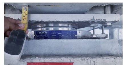
Installation of a RESTON®POT bearing to support the T-beam superstructure of the depot
