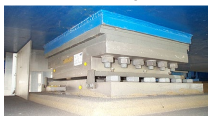
Installed horizontal force bearing
