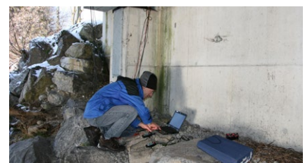
Installation of the ROBO®CONTROL automated monitoring system
