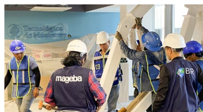
mageba technicians were on site to supervise the installation of the dampers
