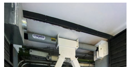
An installed RESTON®SA shock absorber in the campus building
