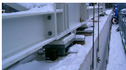
The bearing as a connecting element between the roof construction and concrete
