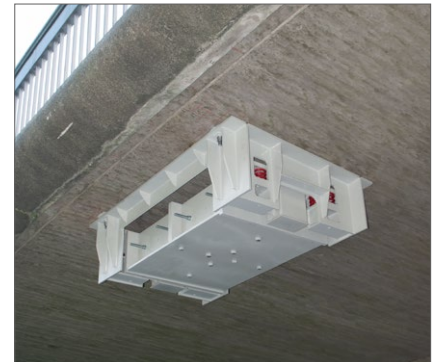
Tuned mass damper with a natural frequency of 4.3 Hz and a mass of 3.5 t, installed on a bridge in Kiel, Germany
