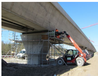
When a bridge bearing requires to be replaced, the costs (including for lifting of the bridge deck) can be substantial
