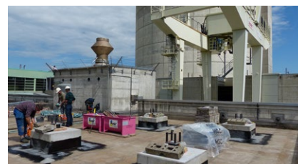
Installation of the LASTO®LRB lead rubber bearings on site at the power plant
