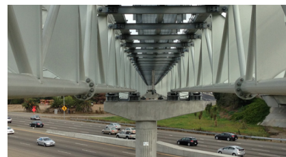
View of four LASTO®BLOCK elastomeric bearings at one pier.
