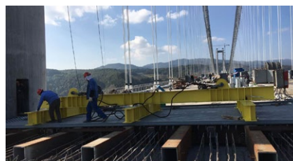
Arrival of the joints with the biggest movement capacity ever (1,920 mm, +/-350 mm)
