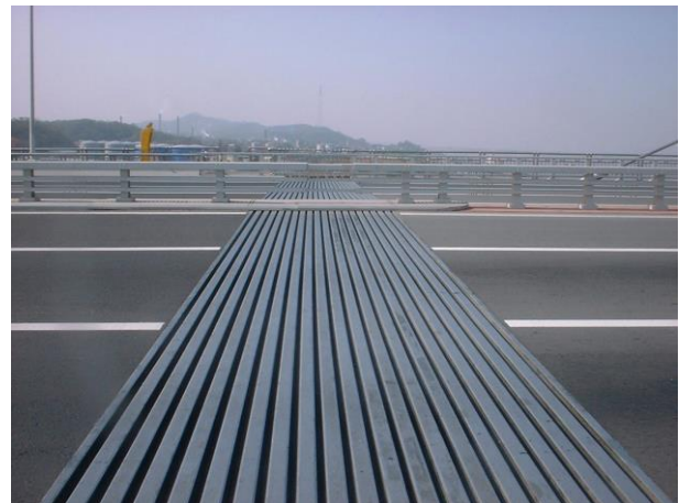
Figure 1. A modular expansion joint, viewed from above, showing the centerbeams and edgebeams that form its driving surface
