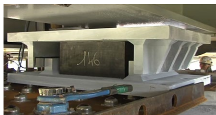
Lead rubber bearing installed in the bridge – guided type, allowing longitudinal movements
