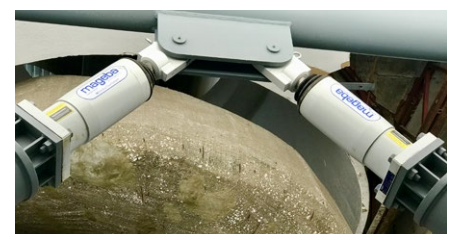
View of one section of retrofitted bracing, with two RESTON®SA shock absorbers
