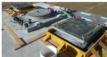
The support of one pier (shear key at centre and a pot bearing at each side) during installation
