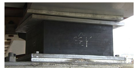
Lead rubber bearing installed in the bridge – multi-directional type, allowing all movements
