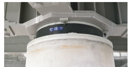
One of the pendulum bearings installed on a column of the building
