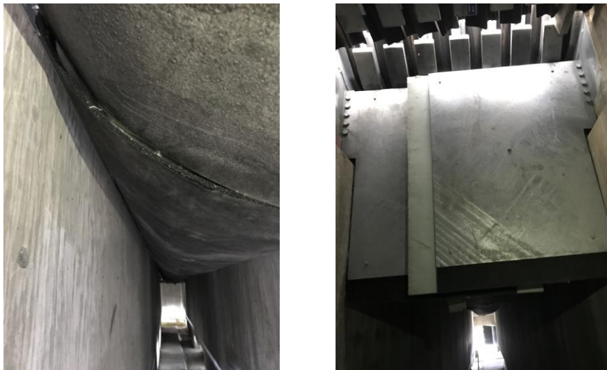
Figure 9. Noise-reduction system applied to the underside of modular expansion joints of the SR520 West Approach Bridge, Washington.
