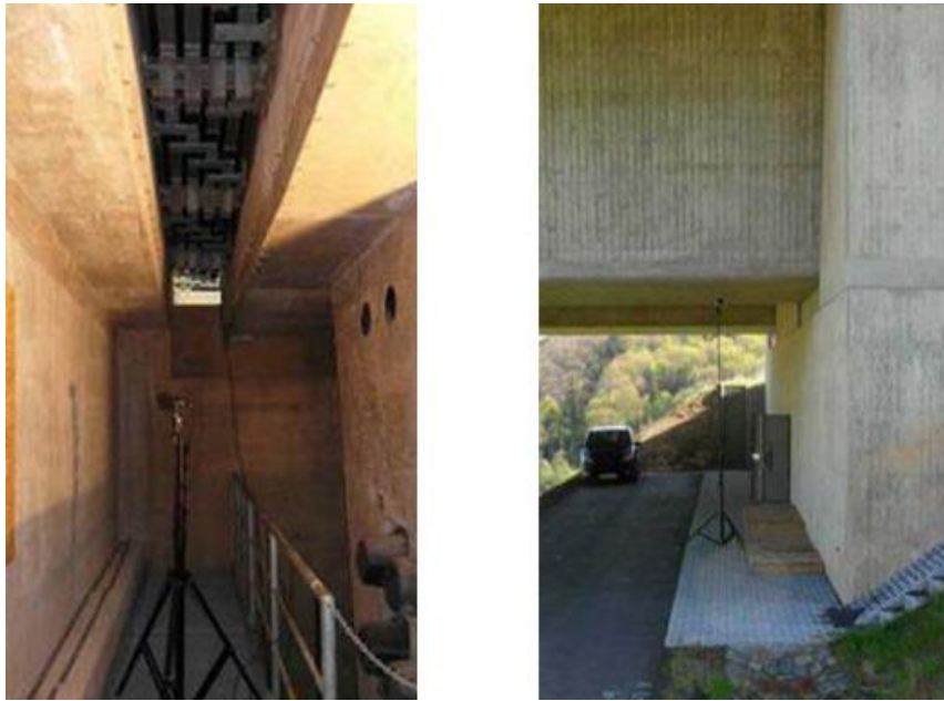
Figure 10. Measurement of noise under traffic of specified types/speeds, both inside the bridge abutment beneath the expansion joint (left) and outside the abutment beneath the superstructure (right).
