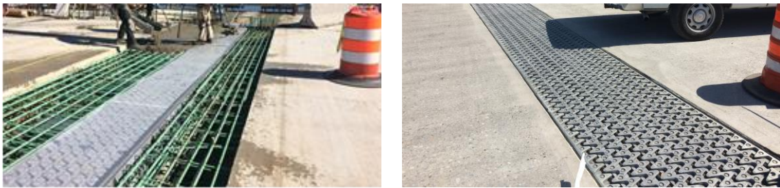
Figure 6. Installation of noise-reduced modular joints of the SR520 West Approach Bridge, Washington.
