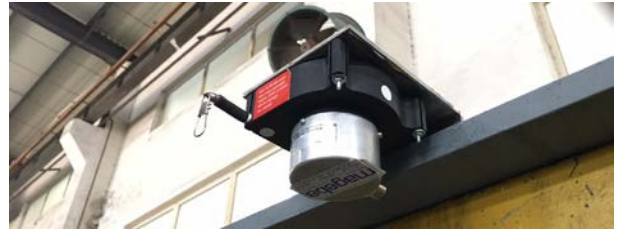
Figure 19. An analogue encoder with cable pull / magnetic sensing for monitoring of longitudinal movements
