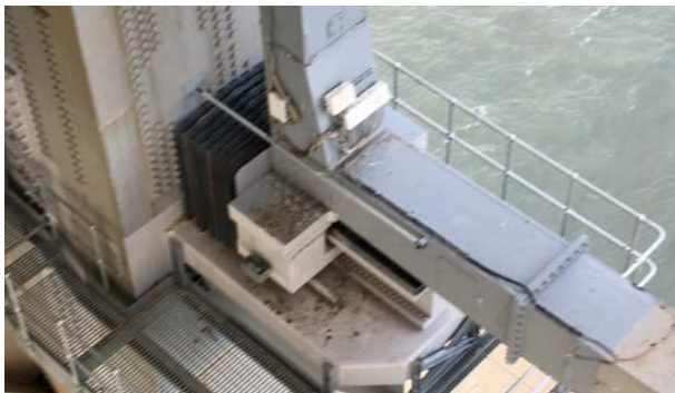
Figure 11. Completed solution, with new bearing installed and supporting the deck truss. One end of the bearing's T-beam, at the tower, is enclosed in a protective expanding/contracting shroud
