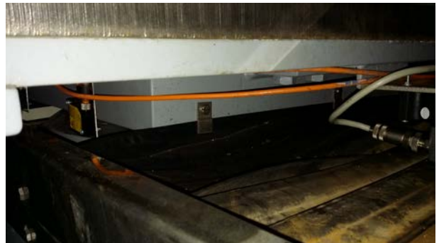
Figure 20. Following installation, connection of a bearing's integrated sensors to the bridge's existing SHM system by means of suitable cabling
