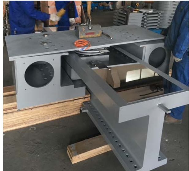
Figure 15. Placing of top plate with uplift clamps hanging down around the T-beam's top flange
