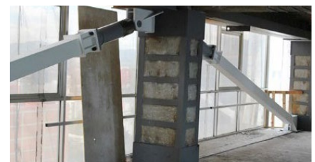
The seismic protection solution with retrofitted steel bracing featuring RESTON®SA shock absorbers
