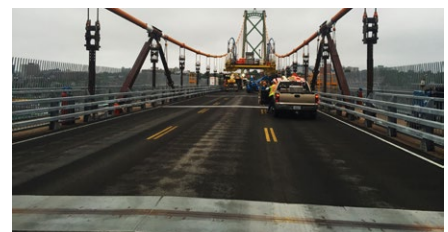
Temporary plates at the point of future installation of the expansion joints
