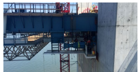
Installed shock transmission unit
