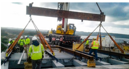
LR20 modular joint being installed on site. Four joints of 10.4 m each were supplied for this project
