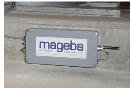
Data acquisition unit of a SHM system
