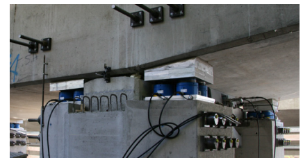
Lifting of deck at one pier using hydraulic jacks on specially constructed plinths at each side
