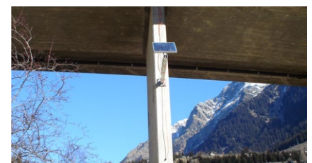
A solar panel on the bridge meets the system's energy needs – ideal in remote locations
