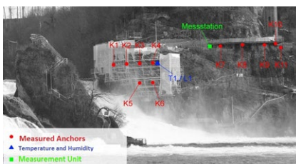
Scaffolding on the cliff face during installation of the SHM system, showing equipment locations
