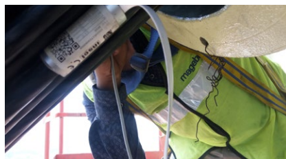
A sensor on a stay cable, measuring high-frequency vibrations (up to 200 Hz)
