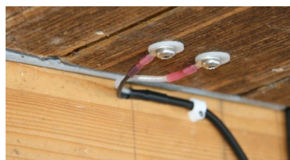
Sensors on the bridge's timber deck measure moisture content
