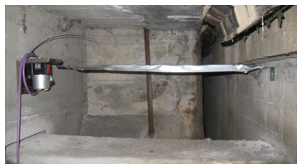
Installed movement measuring sensor with an accuracy of 0.1 mm
