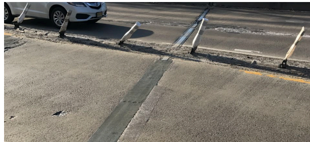
Figure 18: After two years in service on this very busy road, the new joint is still in perfect condition
