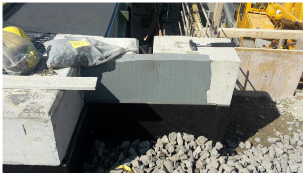
Figure 16: Upstand at end of railway joint following removal of formwork and placing of protection mat (black) and track ballast (stones)
