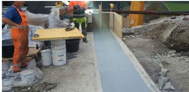
Figure 15: PU flexible plug joint as placed, showing formwork for upstand at one end
