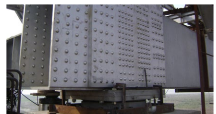
A RESTON®POT bearing as installed, during erection of the bridge deck on top of it.
