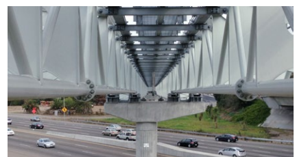
View of four LASTO®BLOCK elastomeric bearings at one pier
