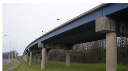
View from below of the viaduct which connects the airport's two terminals
