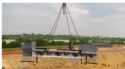
Lifting of a TENSA®MODULAR type LR8-RW joint into position on the bridge
