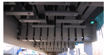
View of a modular expansion joint from beneath, showing its control mechanisms
