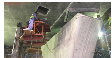
An installed RESTON®POT bearing on a bridge pier
