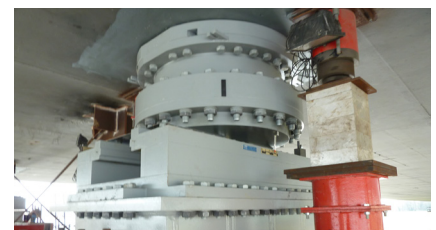
Installation of a RESTON®SPHERICAL UPLIFT bearing (sliding type) under bridge's raised deck
