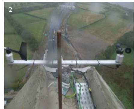
1 Presentation of measured data on web interface 2 Wind sensor as installed on the top of the pylon
