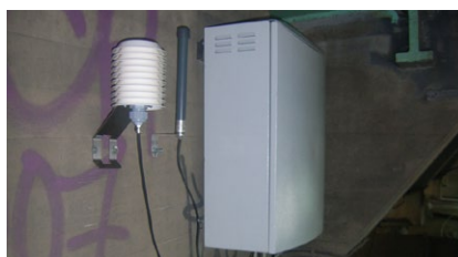
The ROBO®CONTROL Box – the heart of the monitoring system on the bridge
