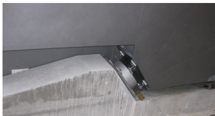
An inclined lifting pot bearing at one end of the bridge
