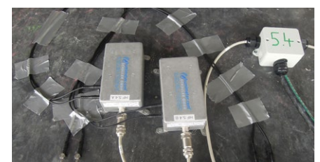
Humidity sensors installed on the underside of the roof
