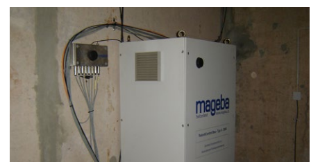
The central computer of the ROBO®CONTROL monitoring system, installed in 2005
