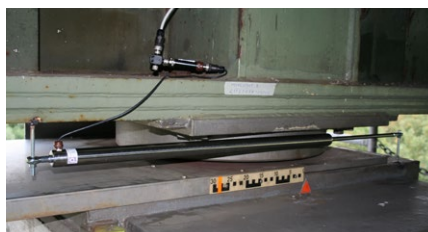
A longitudinal movement measuring sensor as installed at one of the deck’s support bearings
