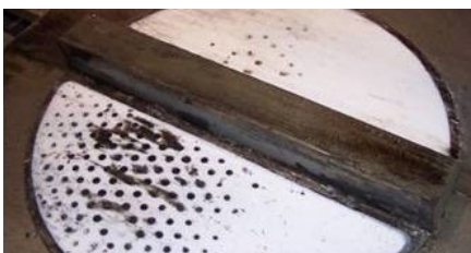
Rapid wear of PTFE sliding discs of the bridge deck’s support bearings required explanation
