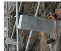
Rock anchor monitoring
